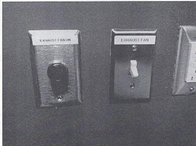
Exhaust Fan Switch and Indicator Light
